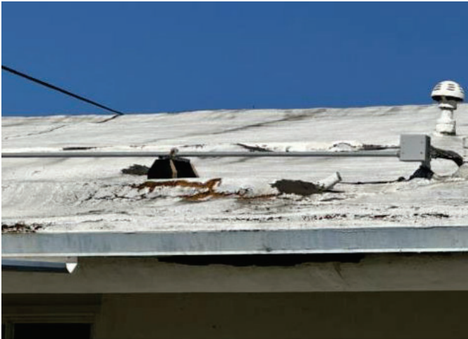
Damage to roof of NUSD district office
